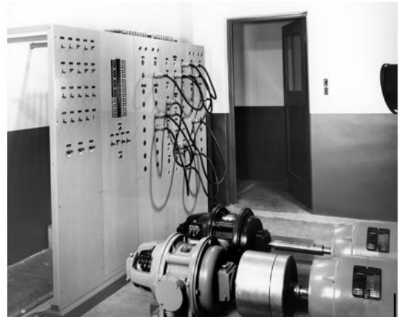
1950s-1970s Interlock generators and patch panel
